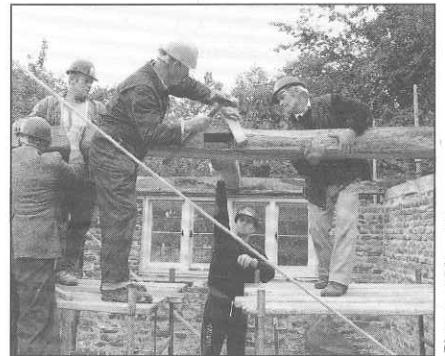
The 16th century timber-framed cross-wing of Longport House takes shape on its new site
